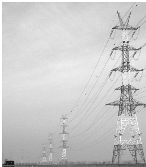
Fig. 1. Rebuilding of a single power line 220 kV to a 4-way power line (2x220 kV, 2x400kV) in Kamionki Borough near Poznan
