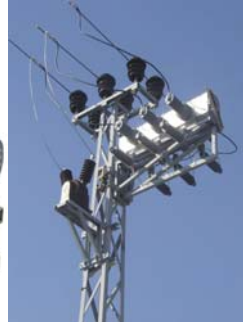
Fig. 6. The figure of NGS at the neighbourhood of Gölbaşı-Şehitali after the installation
