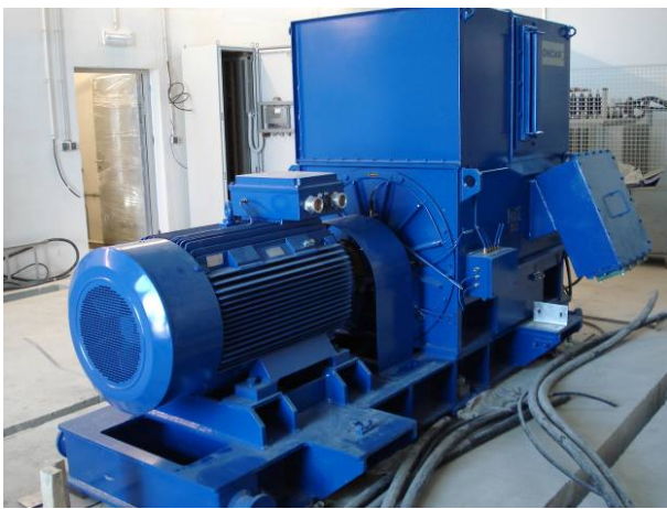
Fig. 6. Induction motor (left) and synchronous generator (right) on site
