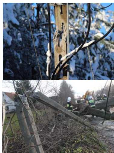
Fig.1. The examples of damages to overhead lines: the ageing of the structure [15], and damages caused by branches of trees [16]
