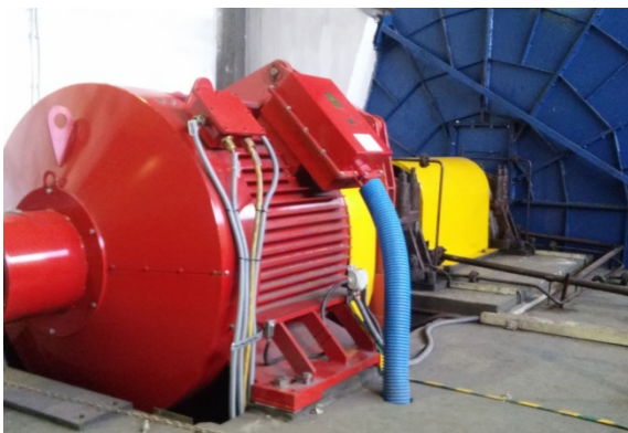
Fig. 8. View of the main fan drive in an underground mine
