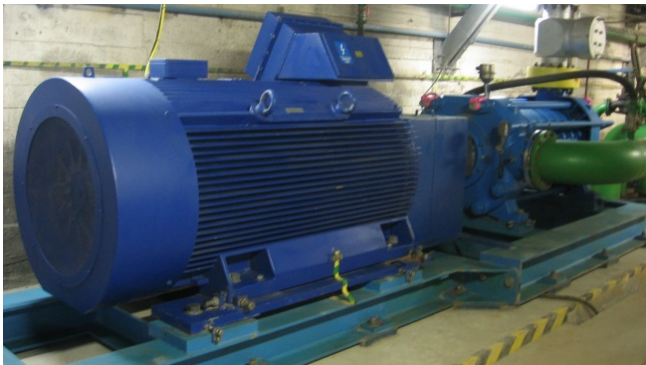
Fig. 6. View of the main drainage pump drive in an underground mine
