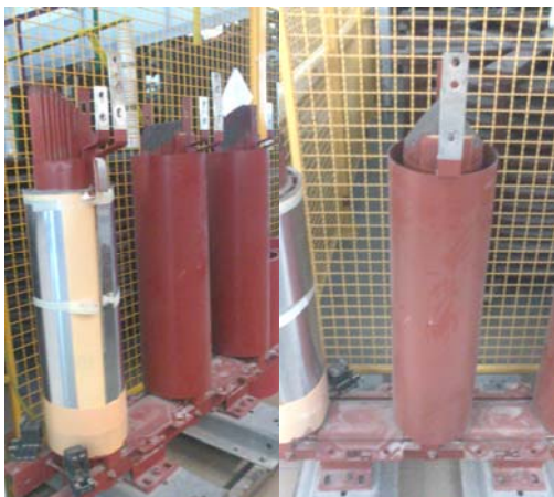
Fig. 2. Picture of TRIHAL transformer without upper yoke
