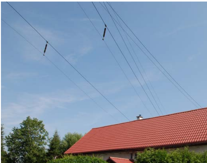
Fig. 1. 110 kV lines with insulators placed between the live line and an additional grounded shielding line
