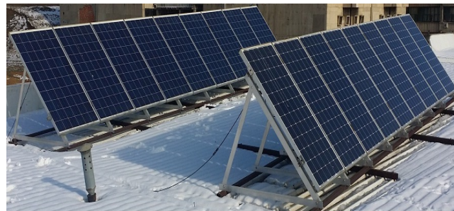
Fig.3. PV modules mounted in the roof
