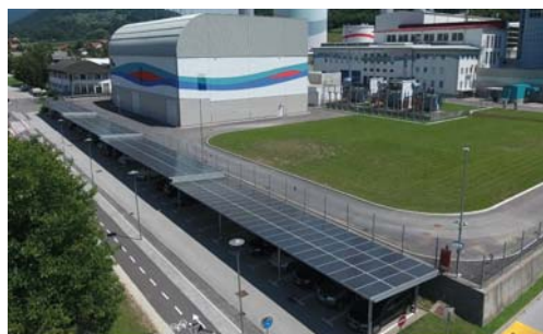
Fig.1. Photovoltaic system installed near thermal power plant Brestanica, Slovenia.
