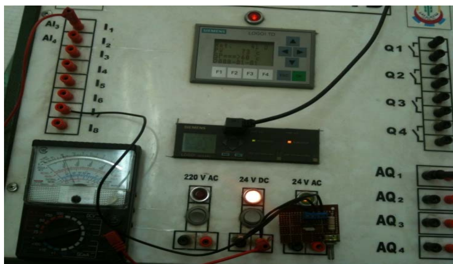
Fig.12. The PLC control board
