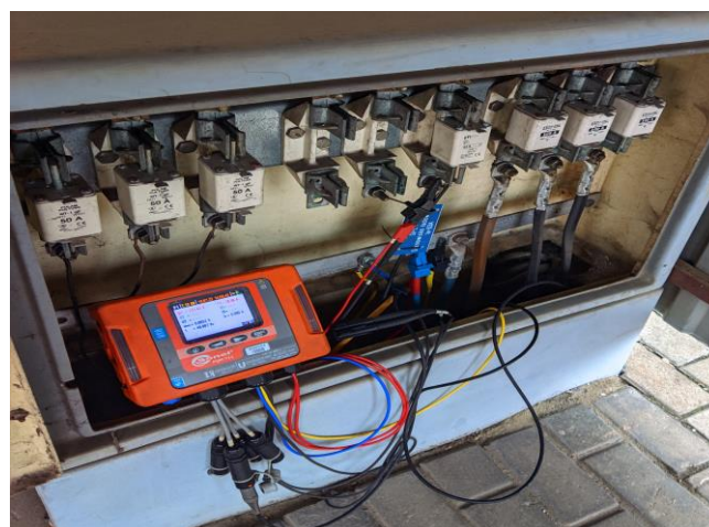
Fig. 1. Setup during measurements of power quality parameters during Nissan Leaf charging at PGE Dystrybucja building in Lublin (Sonel PQM-711 PQ analyser and Sonel F-2 current clamps)
